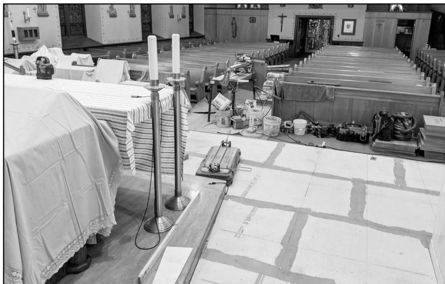
Green carpeting was replaced with ceramic tile at St. Mary's in Waddington. Much of the capital-campaign funded project was completed during the pandemic.
